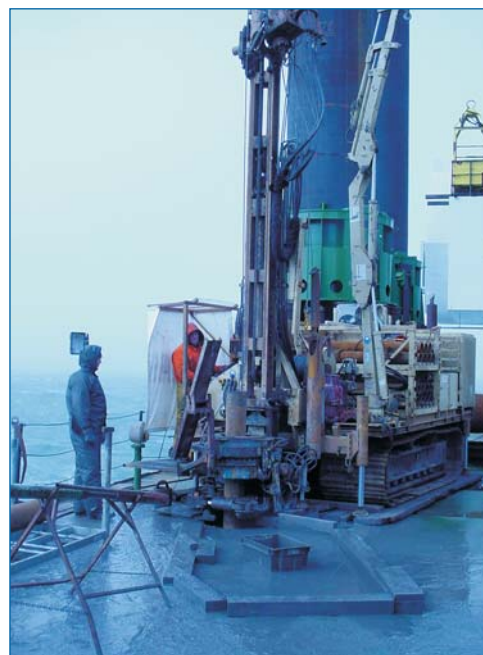
Figure 6 Soil investigation in 2007, drilling in the borrow area from seabed level (>20 m-MSL up to 47 m-MSL) (courtesy PUMA)
