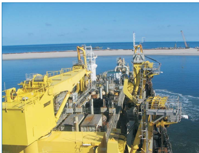
Figure 5 TSHD Oranje, pumping “old” offshore sand (deposited between 100 000–300 000 years ago) ashore via a floating line, and reclaiming the outer Maasvlakte 2 area from sea (courtesy PUMA)
